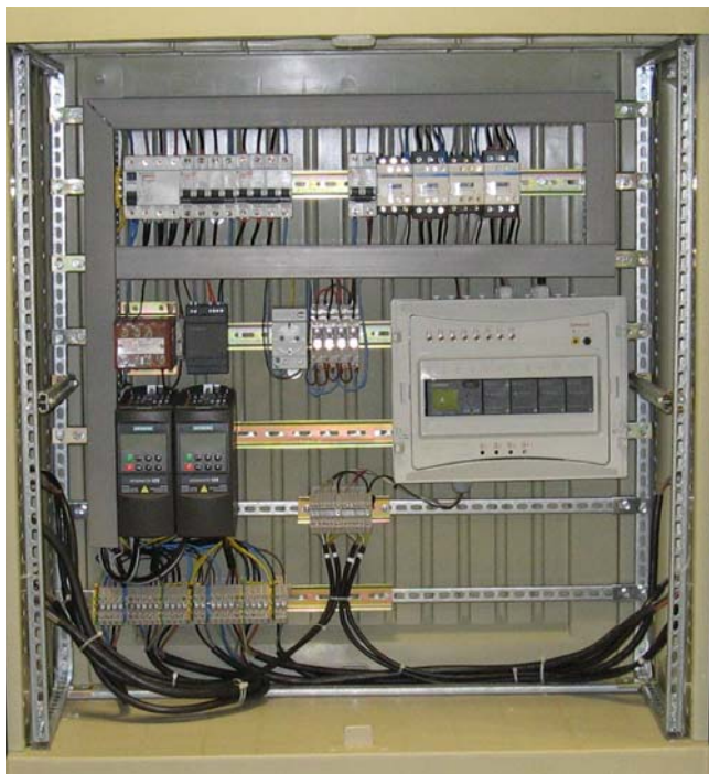
Fig. 6 Control system for automatically controlling of temperature, moisture content and aeration.
